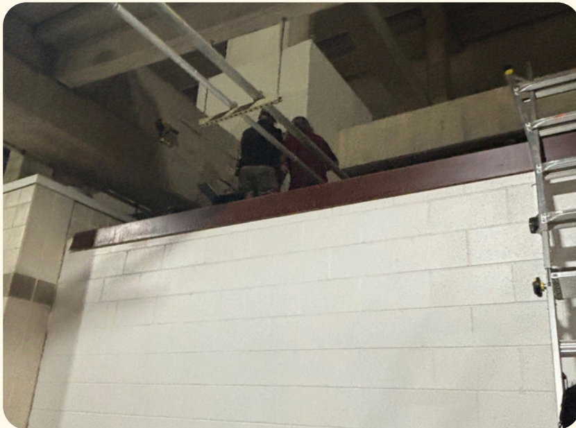
Pictured: Maintenance Services team members Austin Roesler, Brandon Brown, and Glen Gordon respond to the broken main water line during the game.
