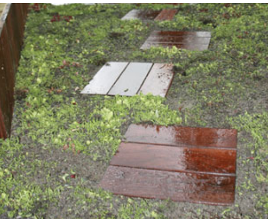
Figure 6. These green-roof panels contain a drought-resistant mixture of sedum and thyme. As the root systems spread, the seams between the panels will disappear.
