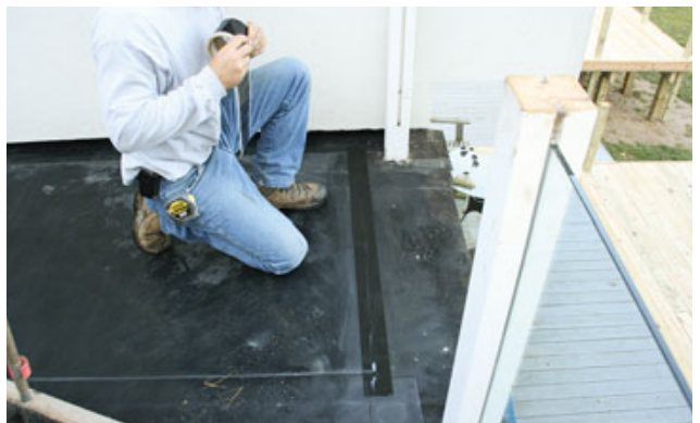
Figure 3. The existing rooftop deck didn't need any structural reinforcement (top), but an additional EPDM waterproofing membrane was installed over the existing one (center). Self-adhering EPDM tape was used at the seams and to seal the membrane to the sidewalls and deck posts (above).
