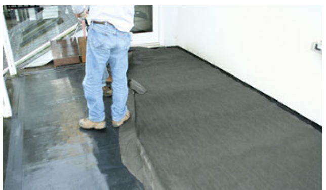
Figure 4. Before installing the deck sections and green-roof panels, workers laid a landscape fabric slip sheet over the waterproofing layer. The slip sheet allows water to drain through and helps protect the EPDM membrane.
