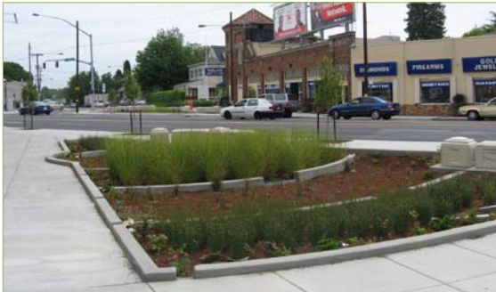
Street retrofits can integrate green infrastructure, like this bioswale along Sandy Boulevard in Portland, Oregon, into standard roadway maintenance and upgrades.
