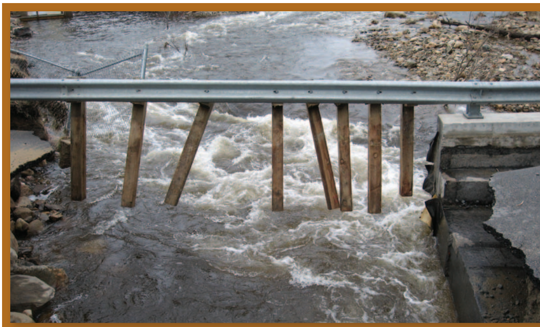
FIGURE 5-2 Mill Pond Road after dam failure at Nottingham Lake, Nottingham, NH, 4/18/2007. Hanging in the picture is the guard rail and support posts for the washed-out road.
