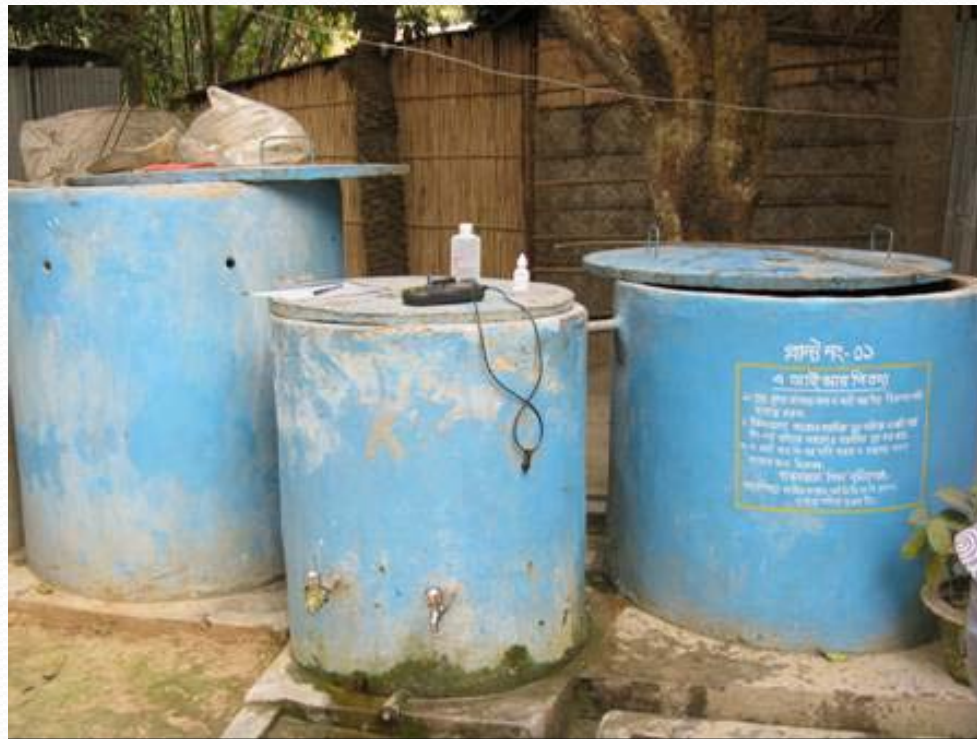
3-Chamber SEDA Plant
