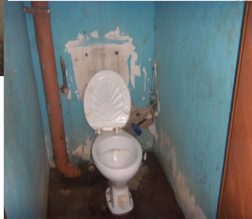
A flush toilet with broken tank
