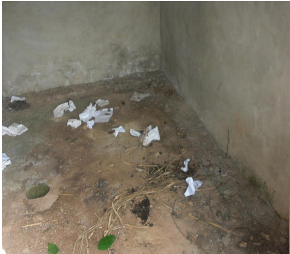
Dirty pit latrine in one of the schools
